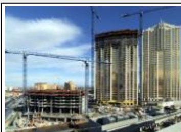
The Residences at MGM Grand are proceeding according to plan as Tower C is at its 7th story and rising.
