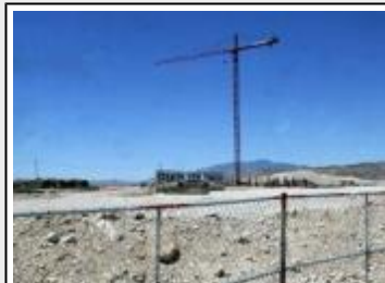
A lone crane sits on the site where Spanish View Towers is scheduled to be built.
